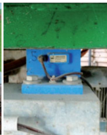
Figure 4 Weighing cell below the feedstock loading unit documents the mass input of feedstock to the digester
